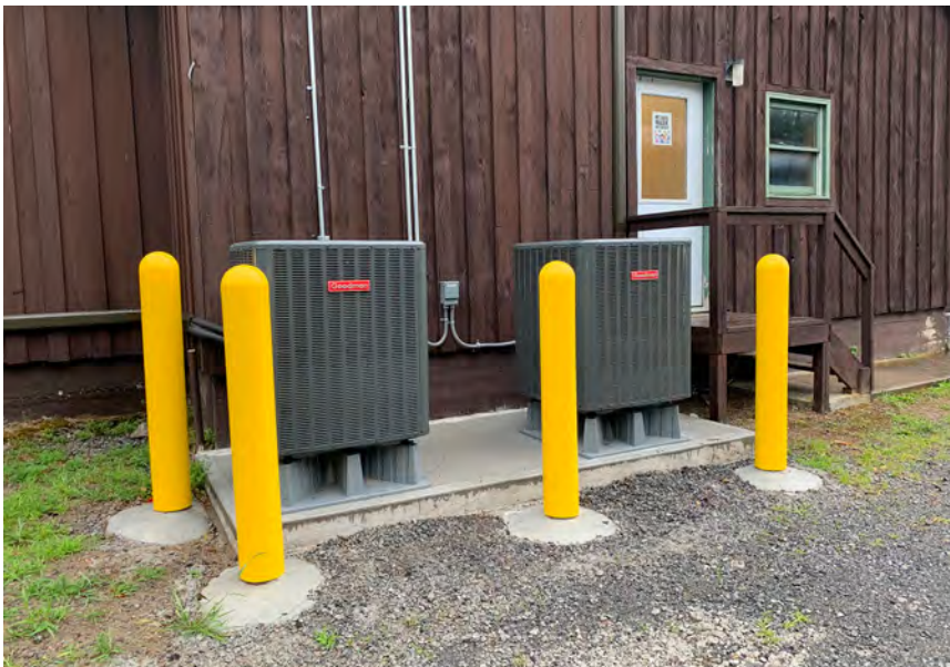
Newly installed Boonville heat pump
