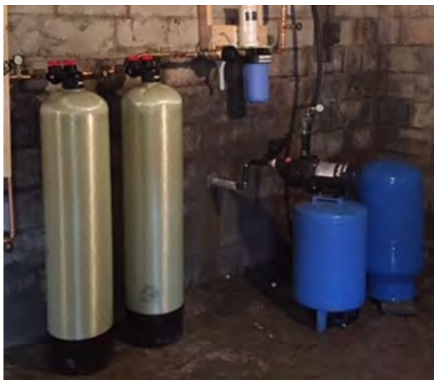
Household point-of-entry water treatment system to remove contaminants
